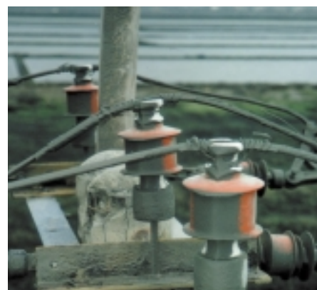
Working conditions of Raybowl insulators
